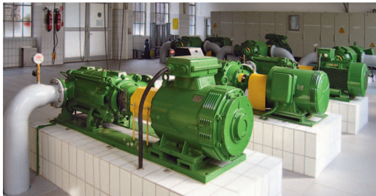
Raw water pipes to aeration tower
